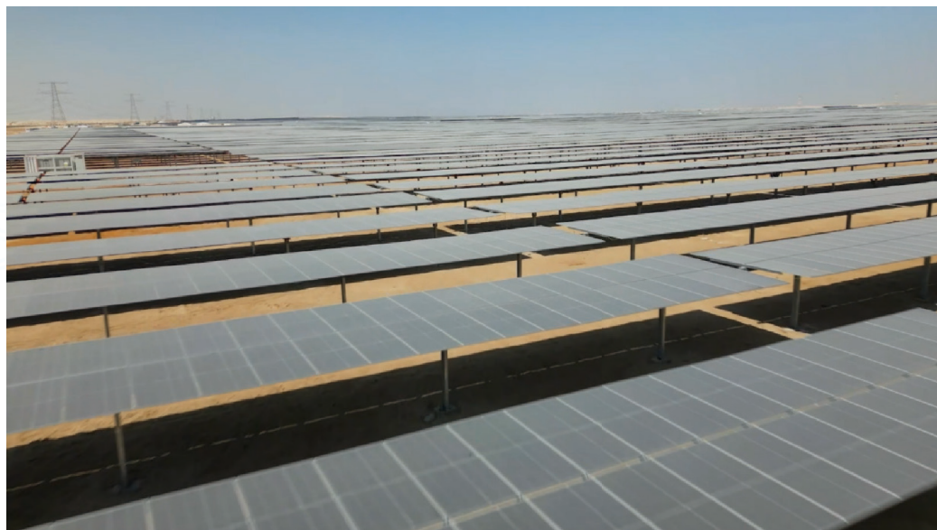
Abu Dhabi Al Dhabra PV2 Solar Power Plant Project
